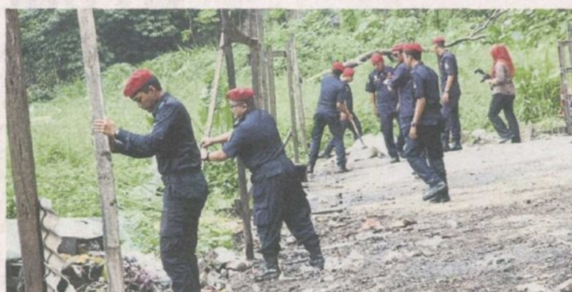
Council enforcement personnel taking down a part of the structure surrounding the dumpsite in Taman Raintree in Batu Caves.
