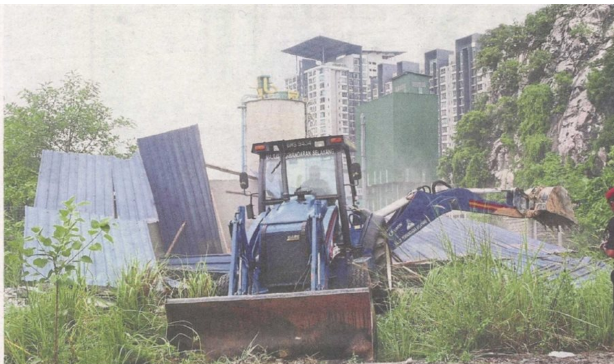
An MPS backhoe being used to tear down an illegal structure during a raid at two dumpsites in Taman Raintree, Batu Caves. — Photos: BRIAN MOH /The Star
